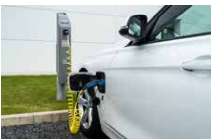
EV charge station with Bender charge controllers inside
